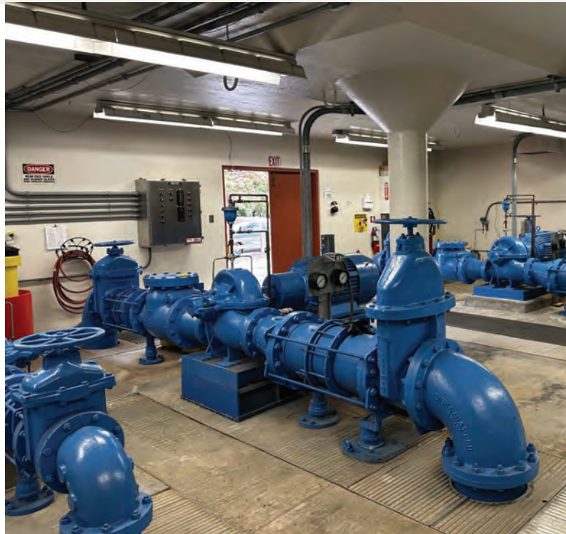
Miramonte Pump Station (Public Works Staff)
