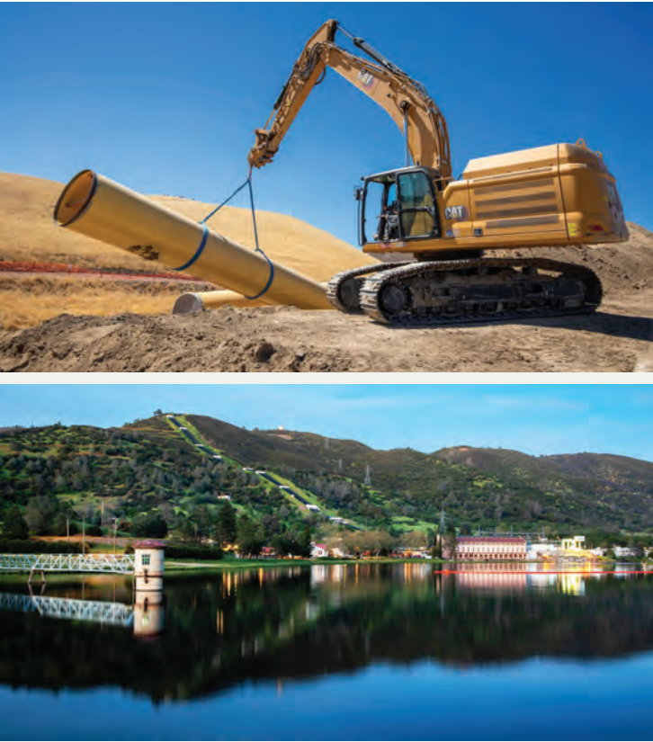
Above, top: San Joaquin Pipeline Valve and Safe Entry Improvements (SFPUC). Above, bottom: Moccasin Powerhouse and Reservoir (SFPUC).
