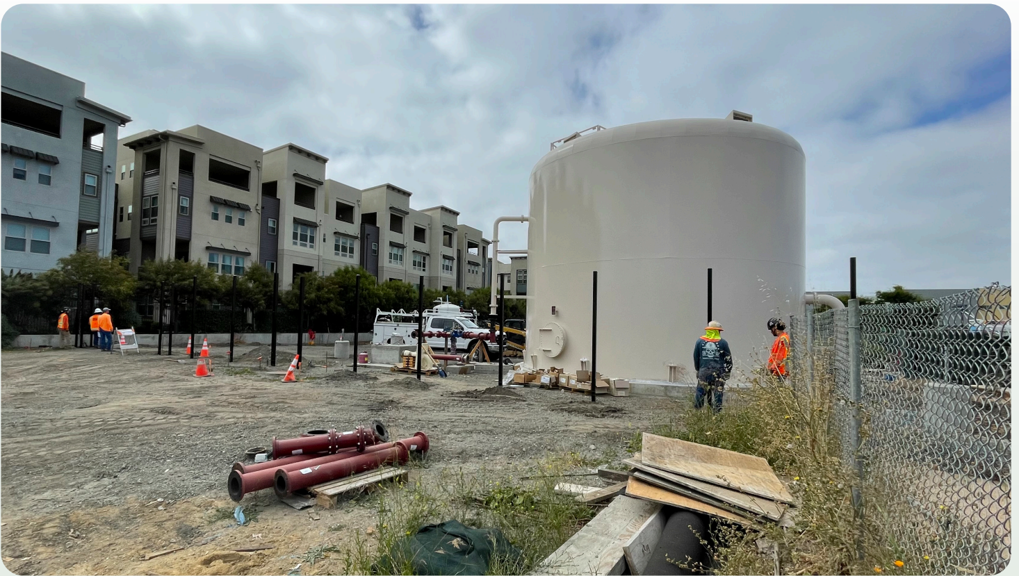
McCandless Well - The McCandless Well will be a production well set to be in operation by 2027. The Well will expand the City's water portfolio, providing a supplemental source of water for City customers.
