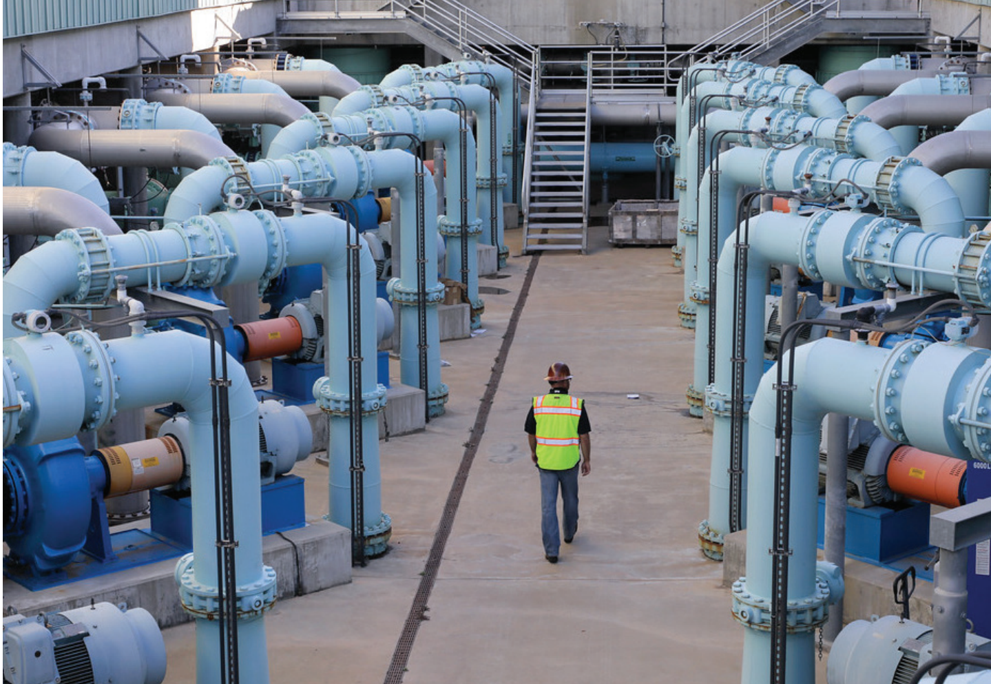
Twin Oaks Valley Water Treatment Plant
