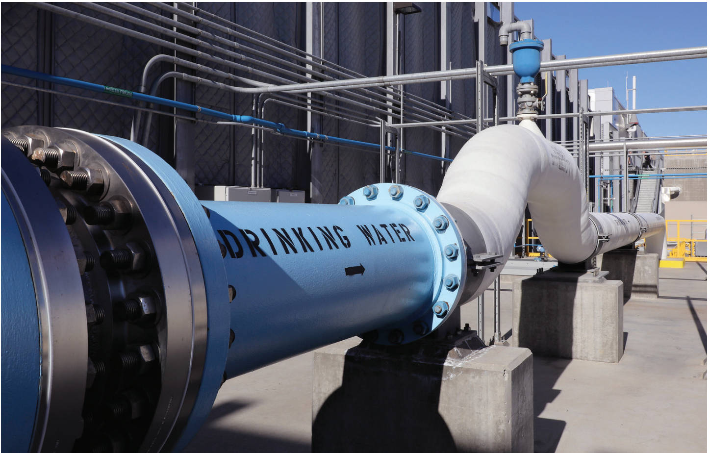
Claude “Bud” Lewis Carlsbad Desalination Plant
