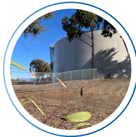
12 Closed Steel Tanks
