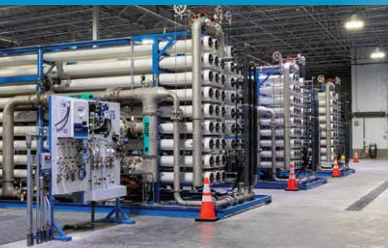
The reverse osmosis system at Pure Water Oceanside. This is where advanced treatment technology helps produce high-quality purified water for the community.
