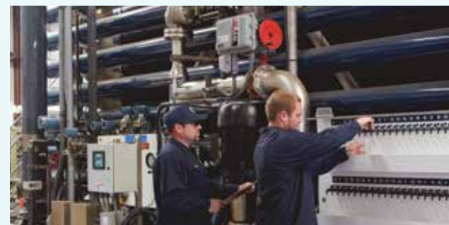
The Mission Basin Groundwater Purification Facility uses reverse osmosis to treat local brackish groundwater extracted from the Mission Basin aquifer.
