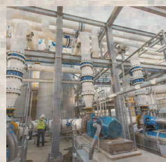
Claude "Bud" Lewis Desalination Plant in Carlsbad
