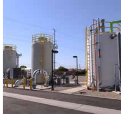
EMWD's Groundwater Desalination Complex provides water for approximately 30,000 homes annually.
