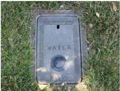
Residential water meter box with a smart meter device.
