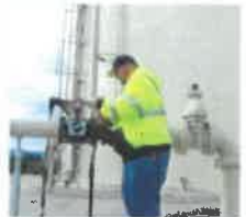
Operational staff regularly operate the automatic air side of the District's reservoirs.
