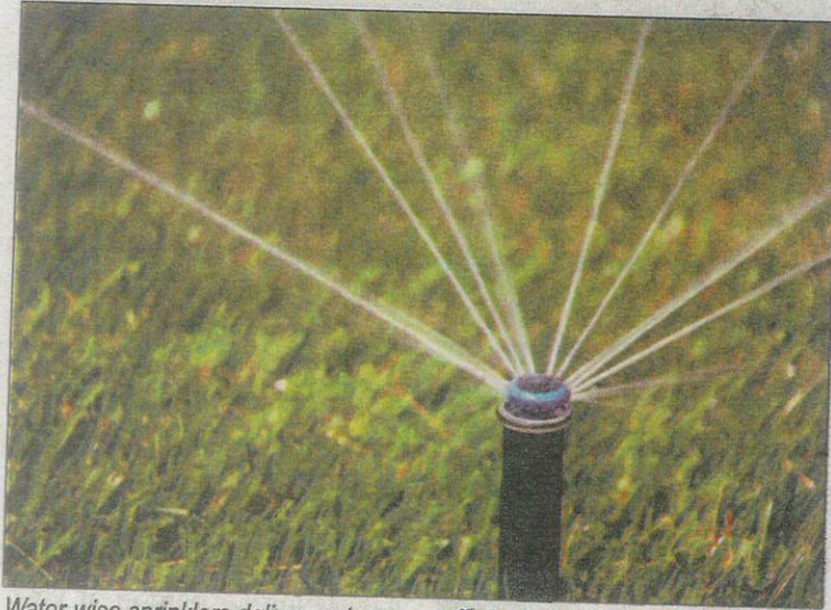
Water-wise sprinklers deliver water more efficiently.
