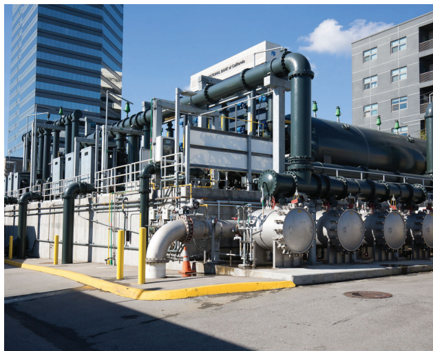
The Arcadia Water Treatment Plant provides multi-barrier treatment to provide safe and high-quality drinking water to the City.
