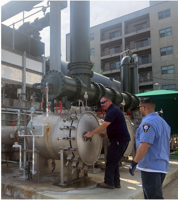
Plant operators perform routine maintenance on the cartridge filters and make sure the system is working properly.
